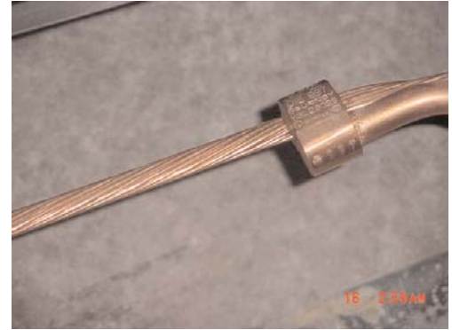
A compression grounding bond.
