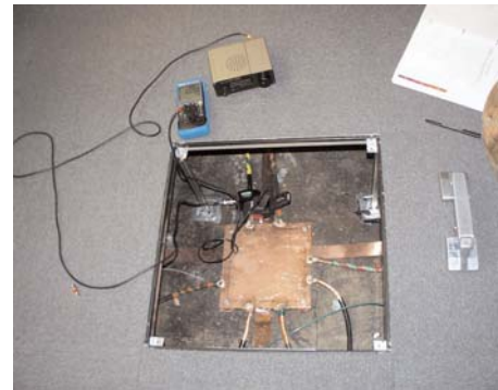
A central ground plate can serve as the common bonding point for many grounds.
