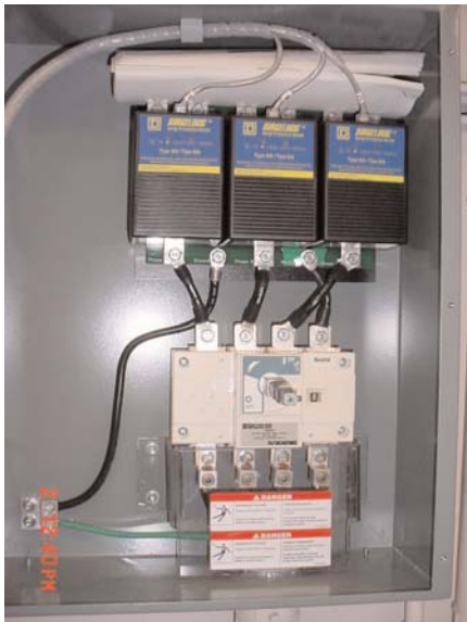
Caption: Surge protection is often installed along with other protected equipment in the same panel.
