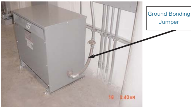
Flexible conduit often requires special accommodations for maintaining good ground continuity.
