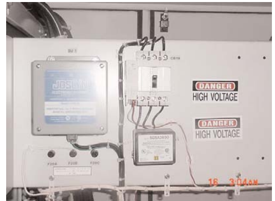
An example of a surge protector installation for a power distribution unit.
